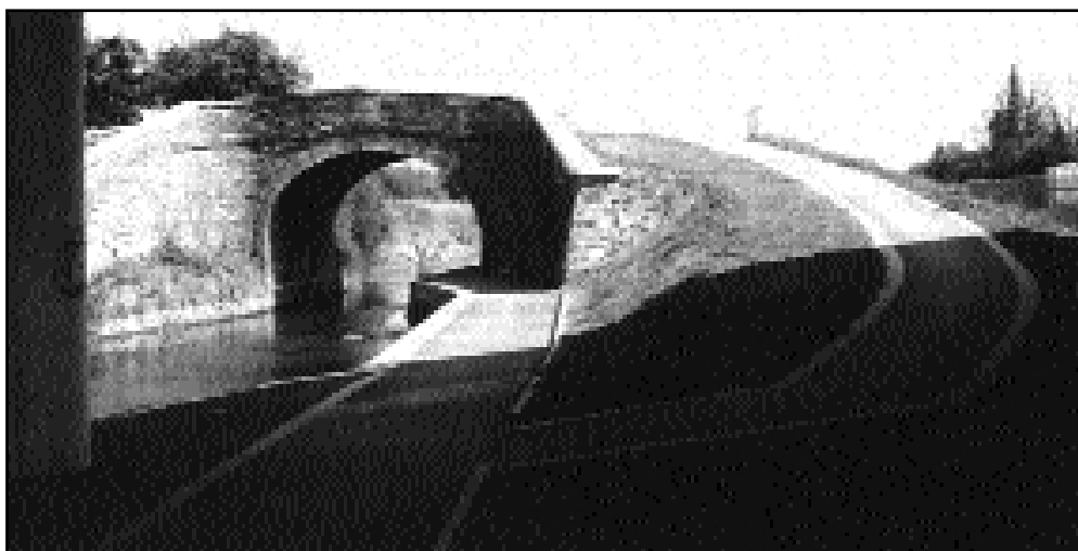
FIGURE 3.25 | ALTERNATIVE ROUTE FOR PASSING THE TUNNEL BY USING THE ENTRANCE TRACK (ON THE RIGHT SIDE) FROM AND TO THE TOWPATH
