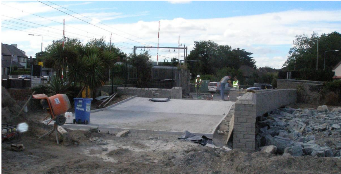
Flood Defence Measures at Merrion Gates
