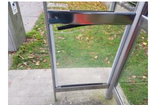
Shelter no 607801 @ University Hospital, Limerick in towards the city. Window glass broken on left hand side of shelter as you look at the shelter.
