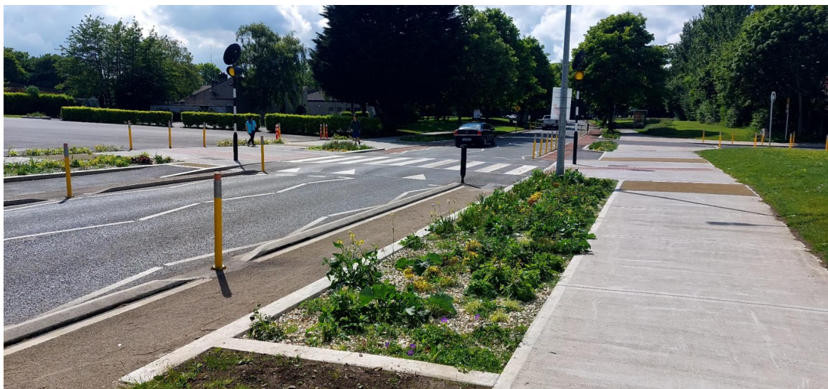
Figure 17 Rain gardens installed in existing verge, footpath widened - Mountview Road, Hartstown, Dublin 15
