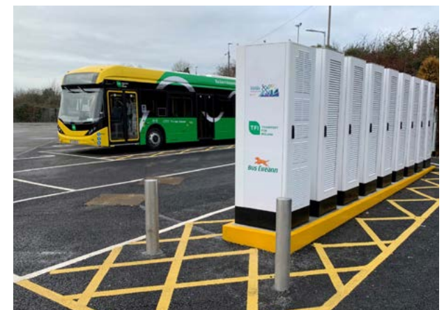
Charging Infrastructure and equipment at Athlone Bus Depot
