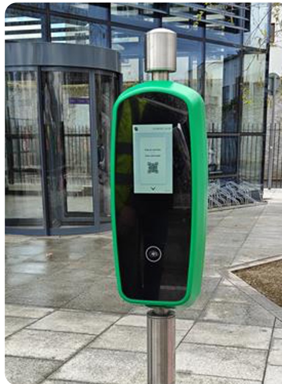
The pole-mounted test validator installed at Broombridge Station
